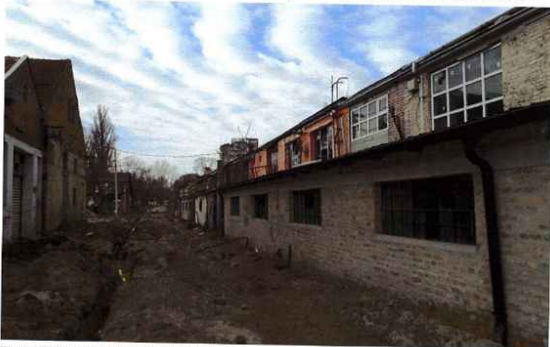
Picture no. 1 Works on the renovation of the facility no. 3 and piping infrastructure.
